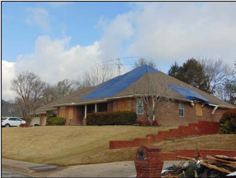
K5YY residence showing window and roof destruction
