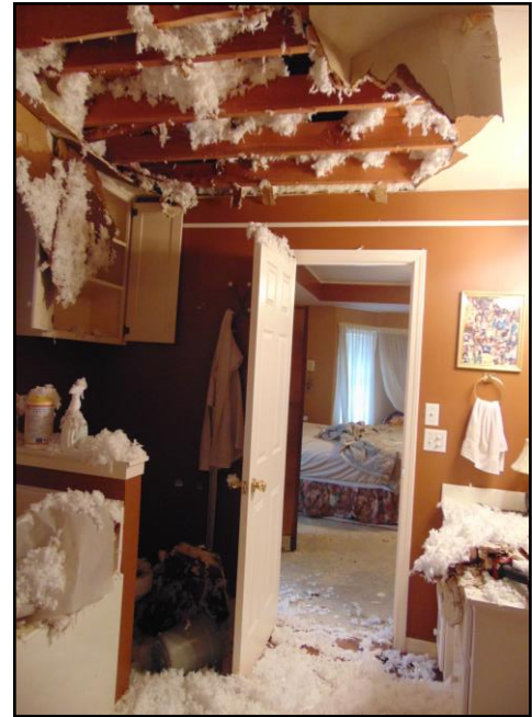
One of several damaged rooms at K5YY
